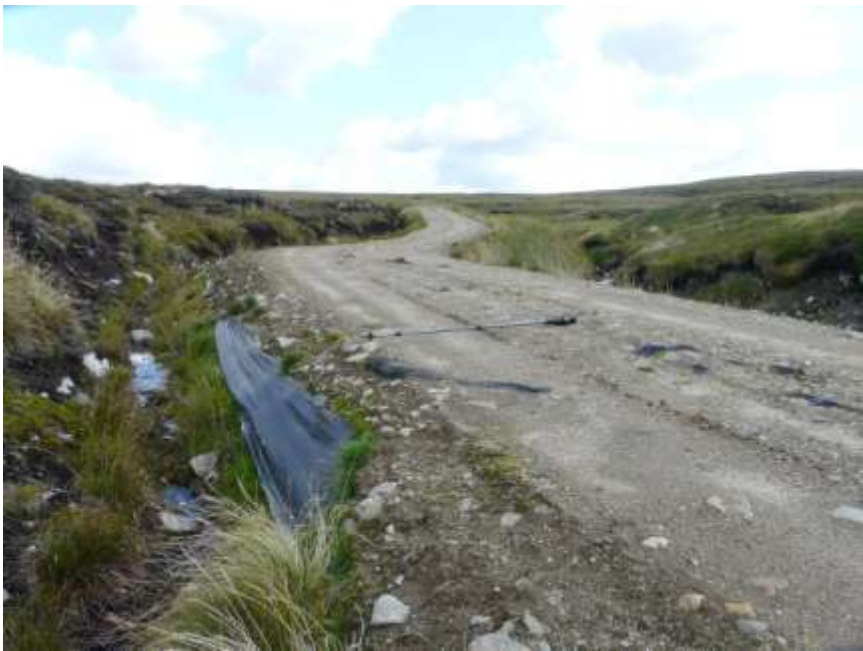
Above: Track eroding off underlying polythene at Kyllachy
