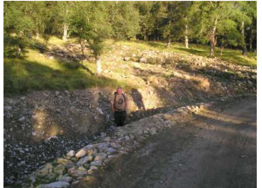
Above: deep ditch and overly steep banks on track in Cairngorms
